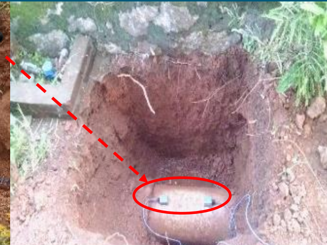
Flow measurement @ OHT common outlet
